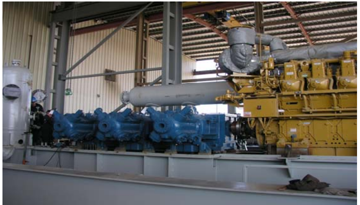
Interconnecting the new engine with the new compression
