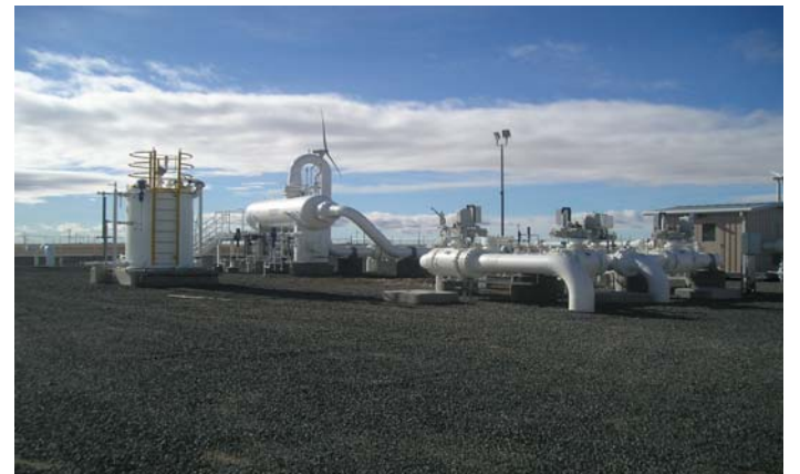
Trailblazer meter station—ECGS interconnect
