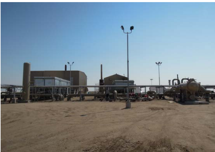
Compressor Buildings and Associated Equipment
