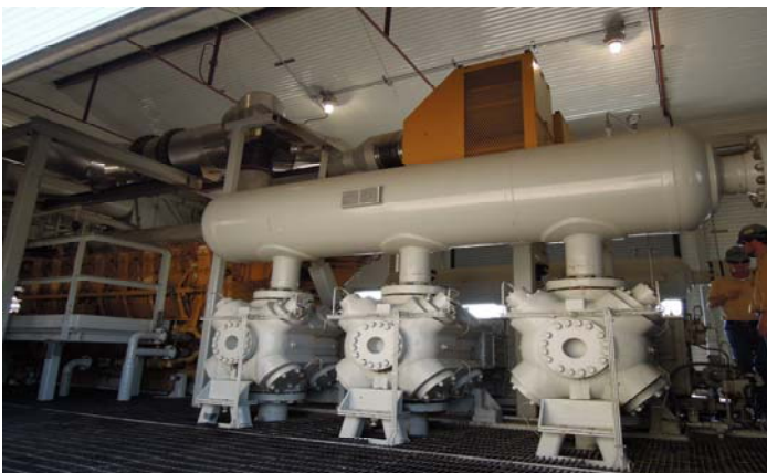
First Compressor and Engine
