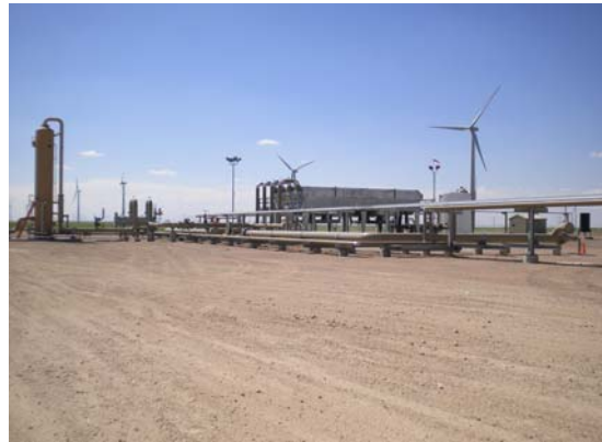
View of ECGS Pipe Racks and Gas Cooling
