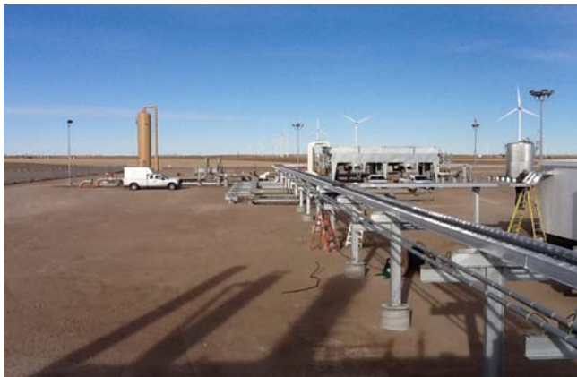
View from the Compressor Station
