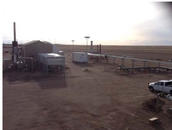
View of ECGS Compressor Station & Piping
